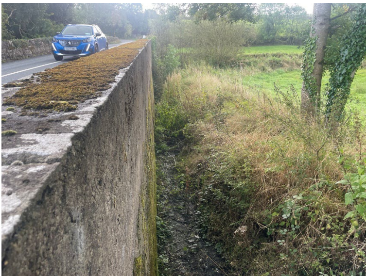
Figure 21 Upstream Bridge wing wall with vegetation growth and section with cement render. View South.
