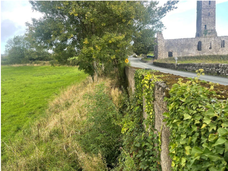
Figure 20 Upstream Bridge wing wall with vegetation growth and section with cement render. View North.
