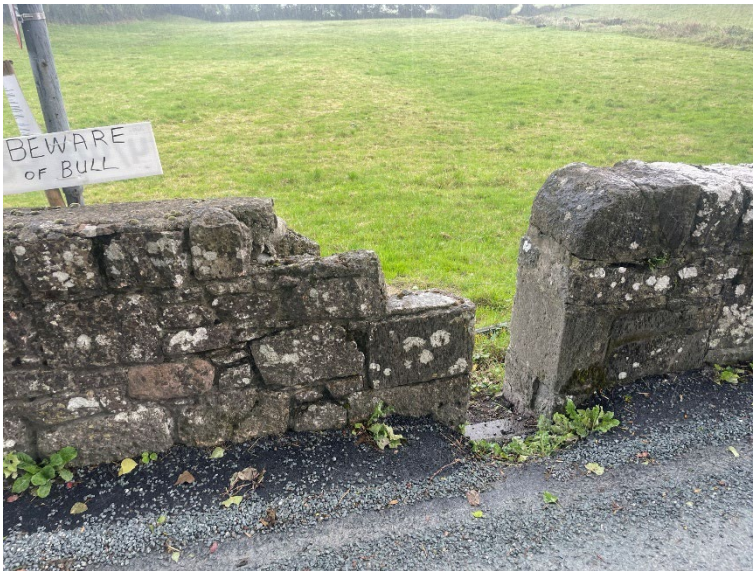
Figure 14 Gap between masonry wall and bridge parapet.
