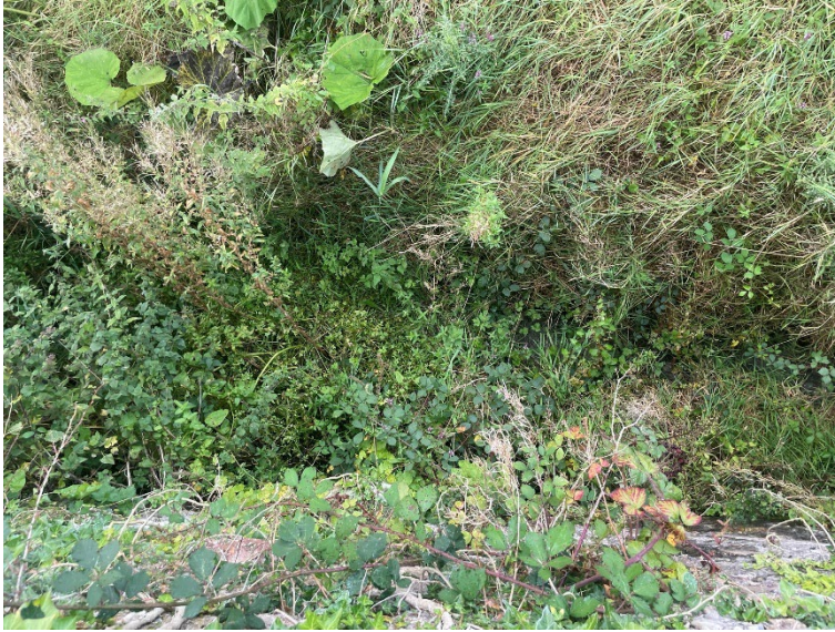
Figure 19 Upstream Bridge Abutment Wall with vegetation growth.
