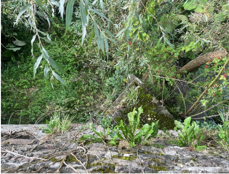
Figure 16 Upstream Ashlar Cutwater (CW-02) with cement render.
