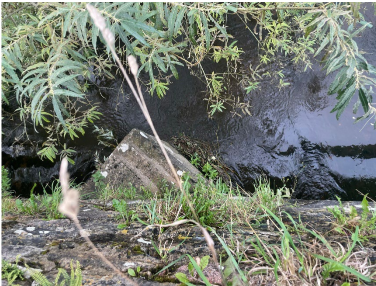
Figure 15 Upstream Ashlar Cutwater (CW-03) with cement render.
