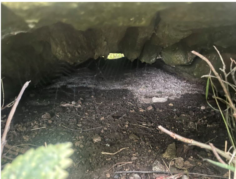
Figure 24 Flood relief arch to the North of the bridge with silt build-up.
